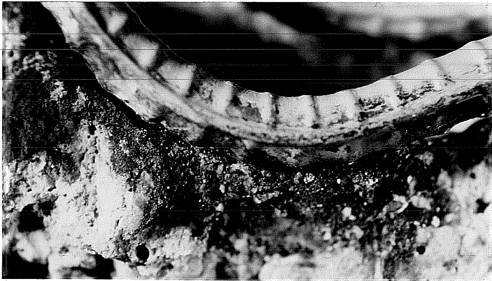
Figure 11.22 Corrosion on Patched Damaged Areas of Stirrup After One Year of Exposure.
