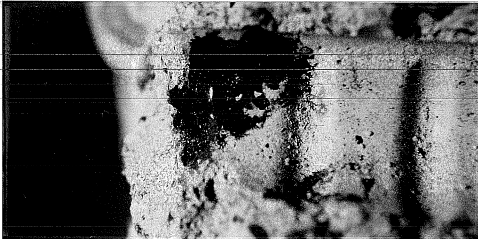
Figure 11.24 Corrosion Spots Coincident with Voids in Concrete.
