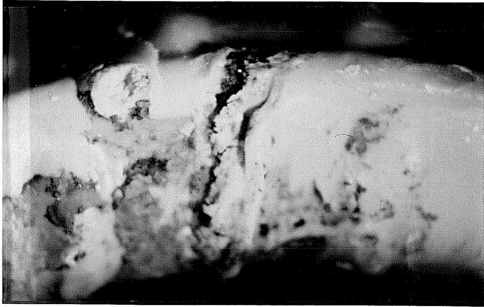
Figure 12.17 Damage of Coating of Stirrup at Contact with Uncoated Bar.
