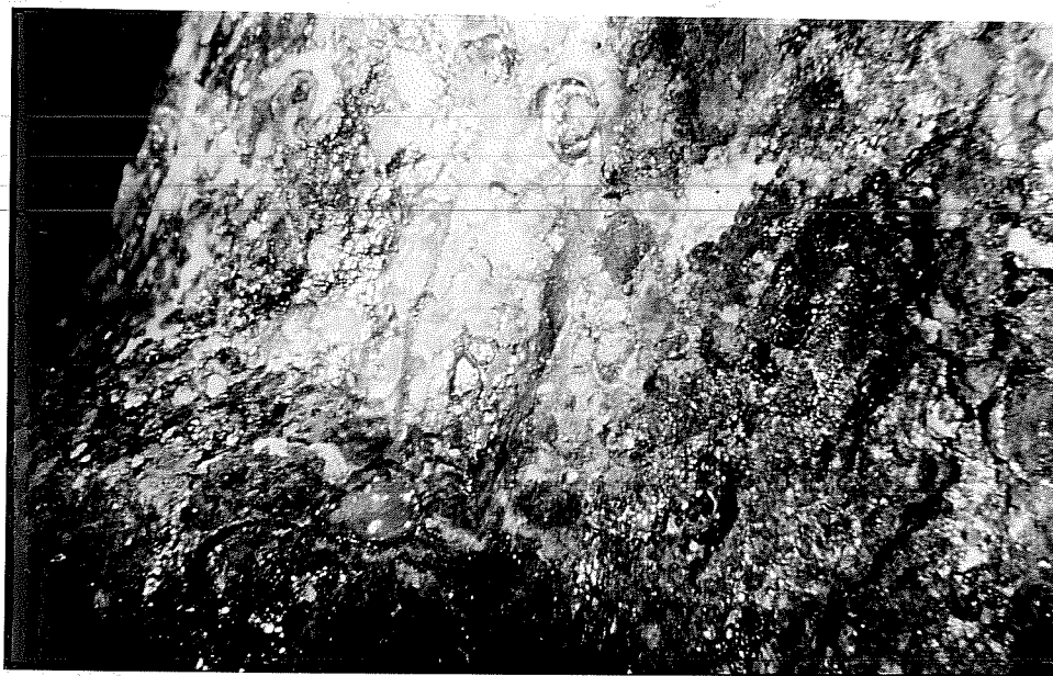
Figure 10.5 Surface Corrosion of Uncoated Bar After One Year of Exposure.
