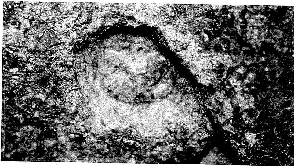
(a) Pitting on Damaged Longitudinal Bar (B11-Upper)
