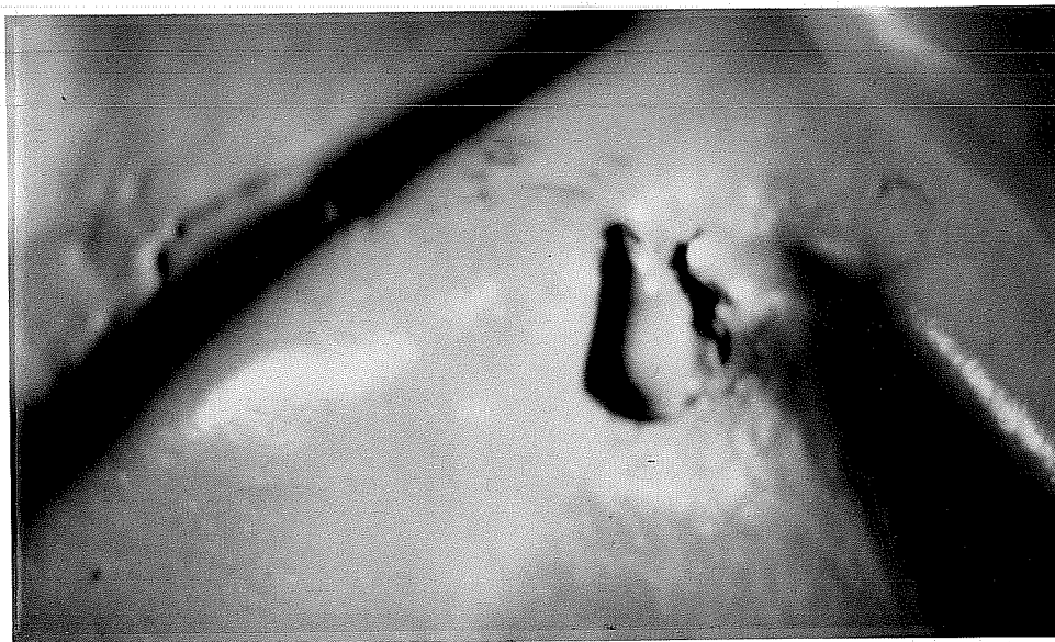
Figure 3.3 Steel Surface Defect at Rib Intersection.
