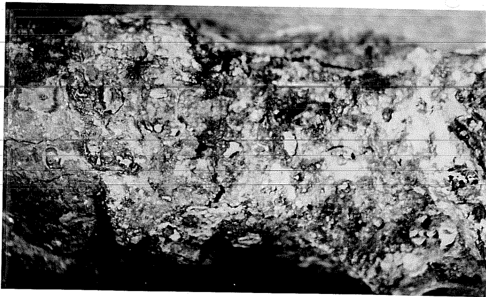
(b) Pitting on Uncoated Bar (B26)
