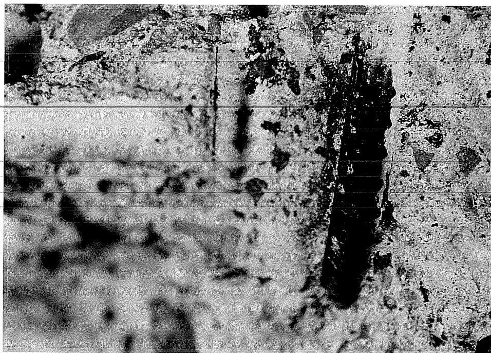
Figure 12.4 Stirrup Trace in Concrete Adjacent to Crack.
