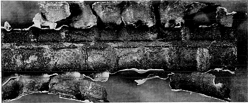
Figure 11.33 Undercutting Along Splice Bar at Patched Cut End After One Year of Exposure.
